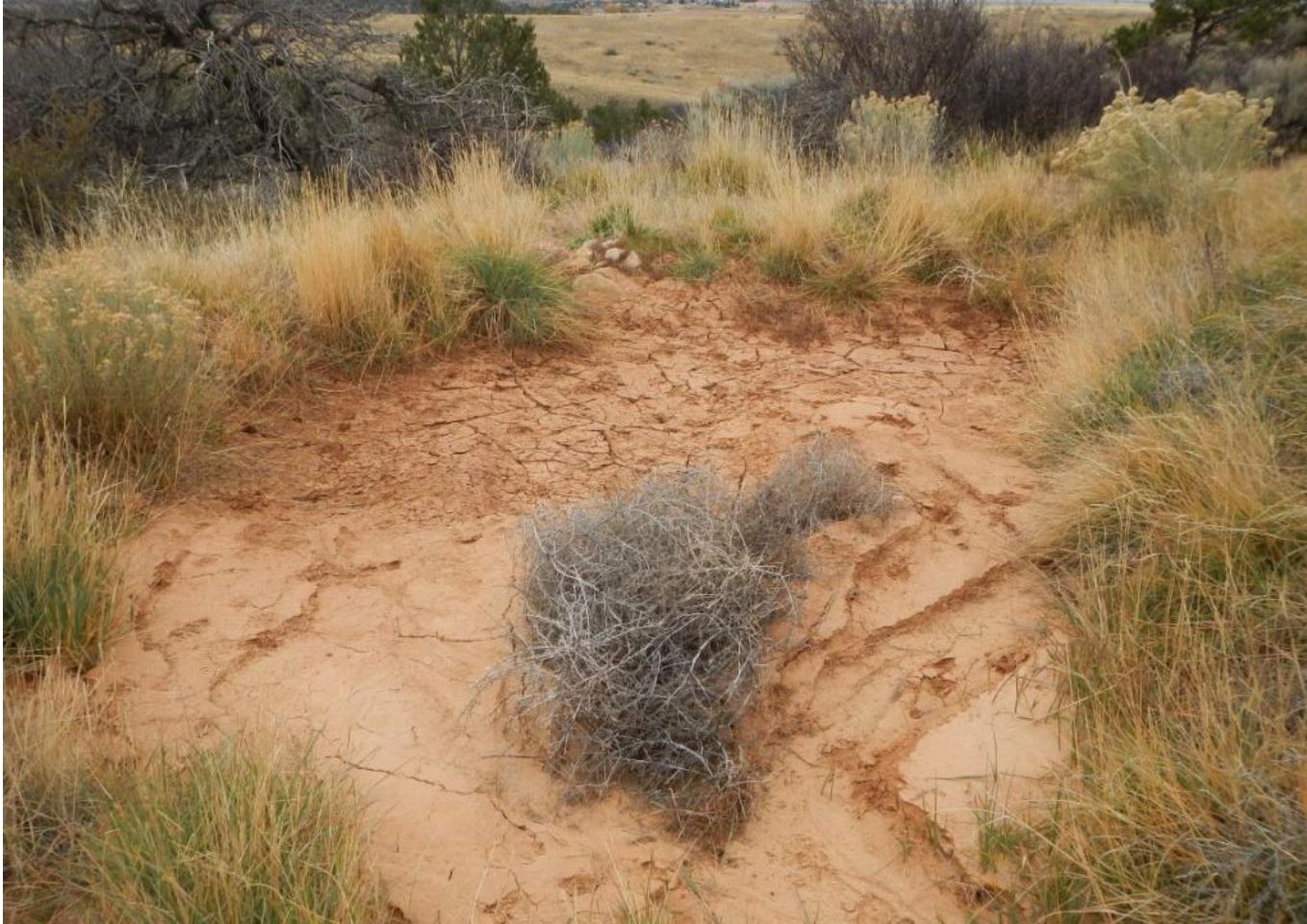
Photo 5. View of silt trap needing to be cleaned out in southwestern corner of project area.
