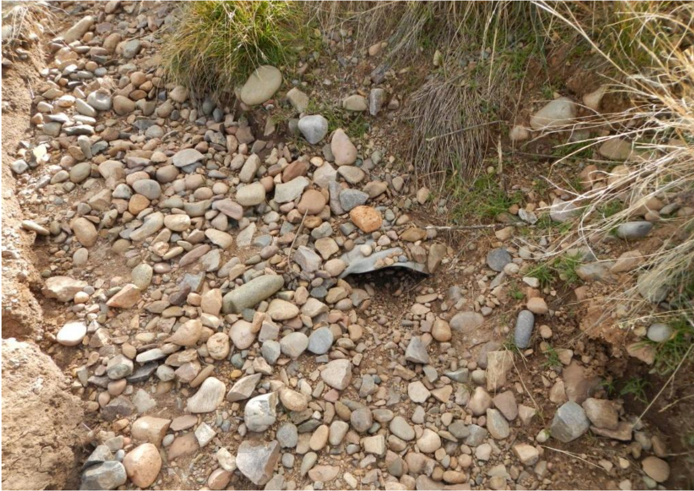
Photo 3. View of culvert outlet at well pad entrance that is full of sediment and rocks.
