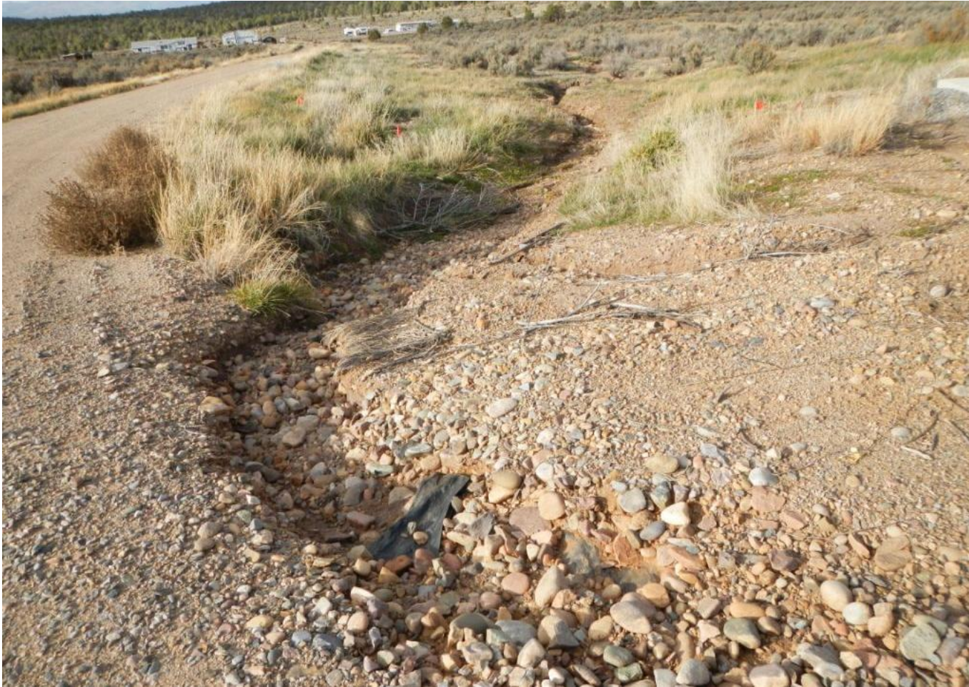
Photo 2. View of diversion drainage (approximately 2 feet wide and 1 foot deep) near well pad entrance that appears to be down-cutting. This drainage should be monitored and BMPs applied if down-cutting/erosion worsens.
