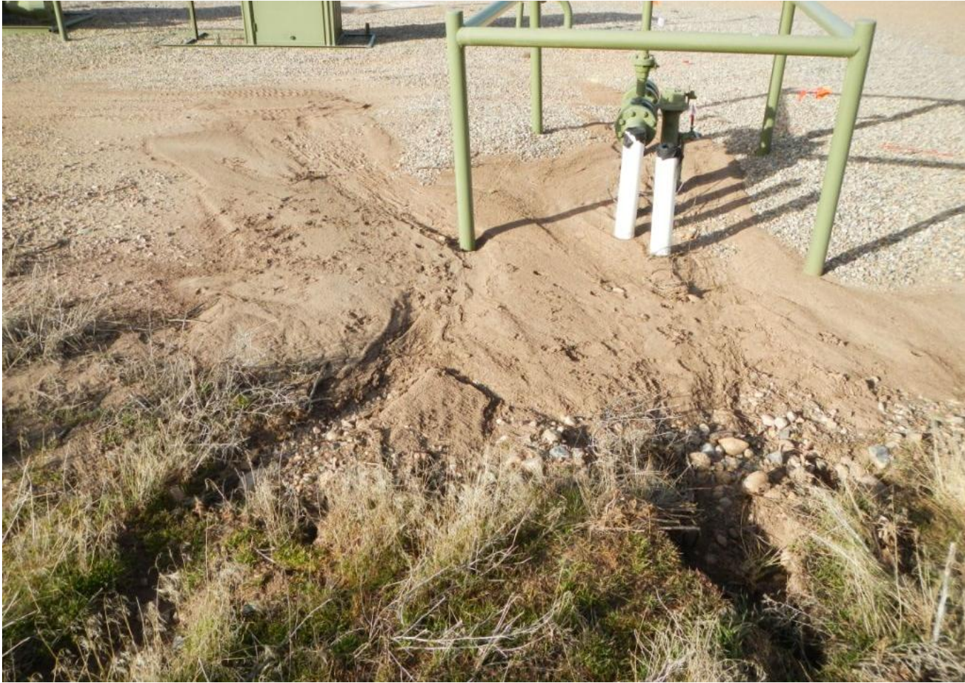
Photo 4. Sediment run-on to the well pad from erosion in the southern portion of the project area. This needs to be monitored and BMPs applied if erosion worsens.
