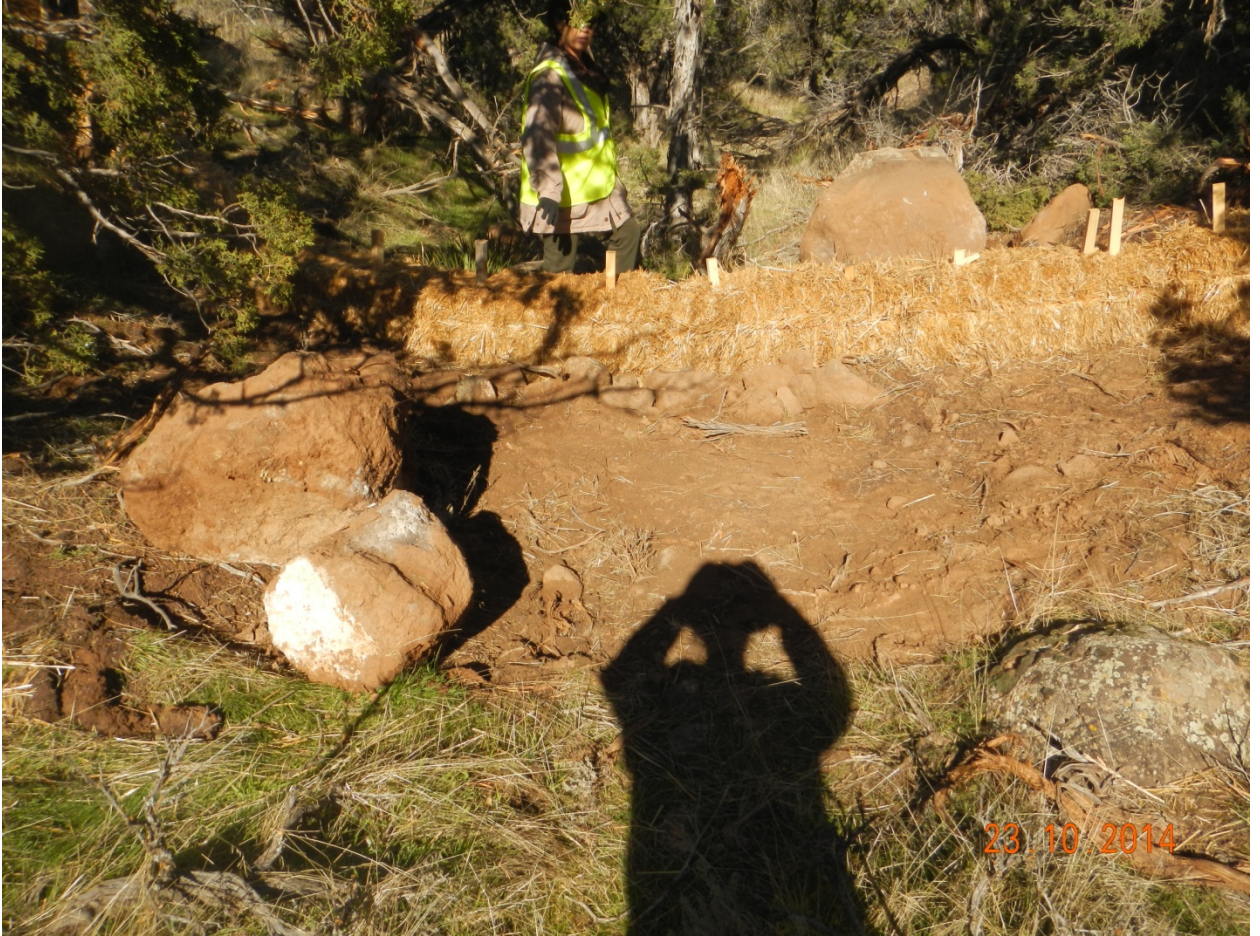
7. Pad Eastern perimeter natural drainage, viewed North from SE quarter along perimeter.
