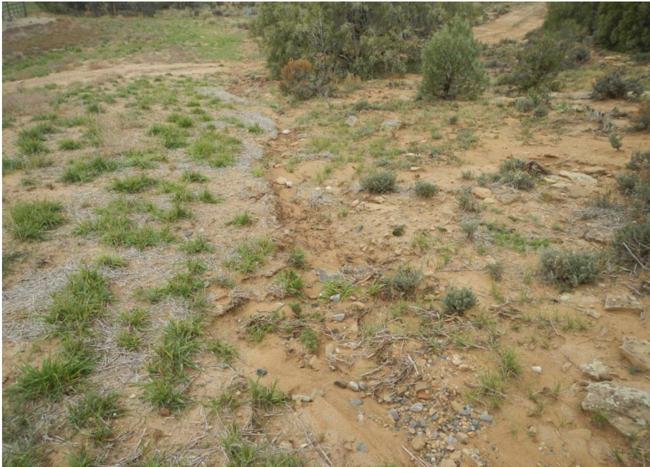
Photo 4. View of erosion from diverted stormwater flows along the northern edge of the project area.
