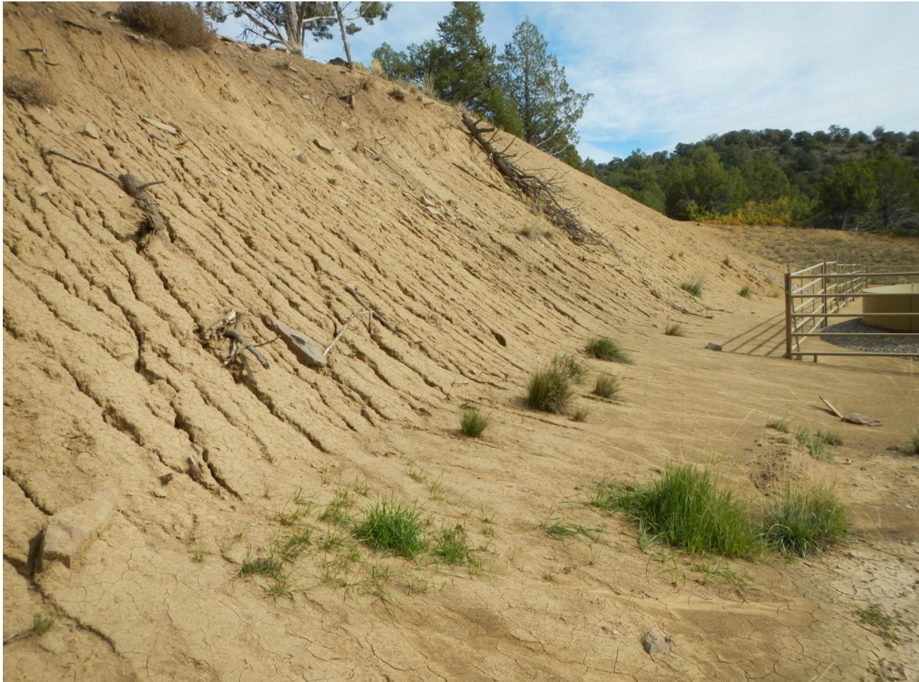
Photo 4. View of rill erosion and sediment run-on along the northern cut-slope for the well pad.
