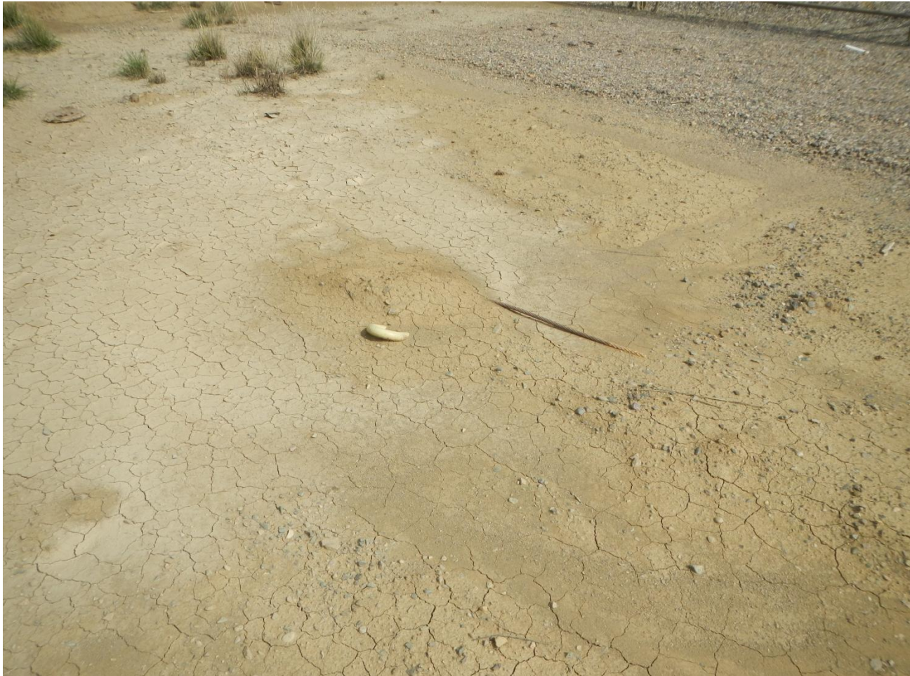
Photo 2. View of partially buried and unmarked guy line anchor as well as partially buried rig cable within the northwestern corner of the project area.
