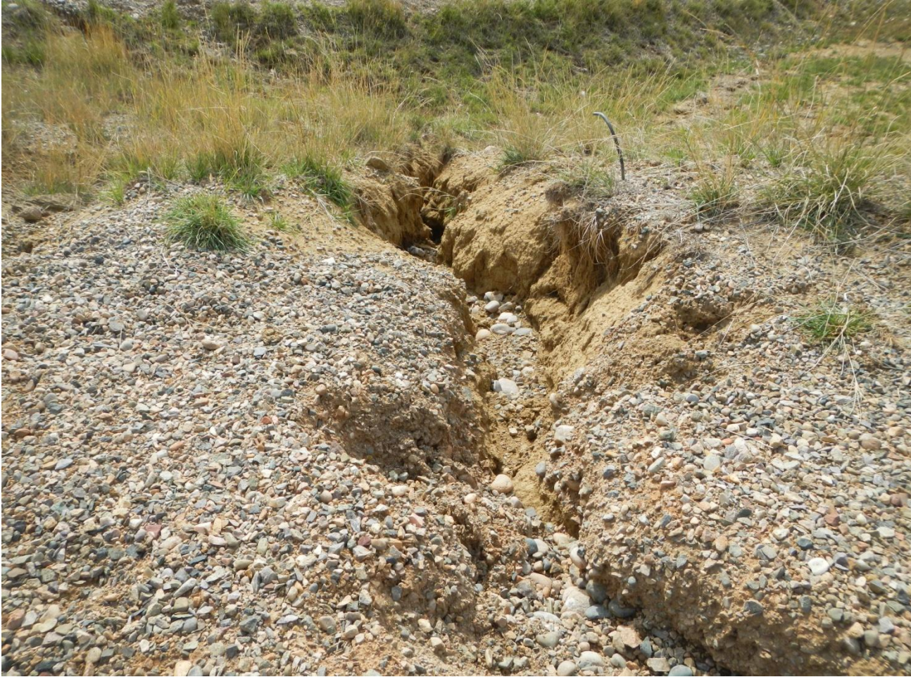
Photo 3. View of gully forming on the southern edge of the well pad near the entrance.
