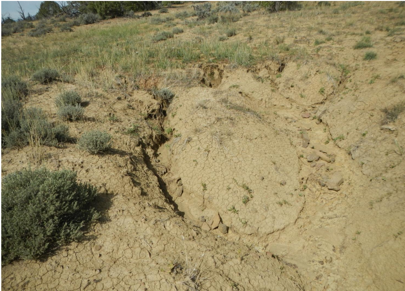
Photo 4. View of more erosion and poor revegetation on cut-slope in western portion of the project area.
