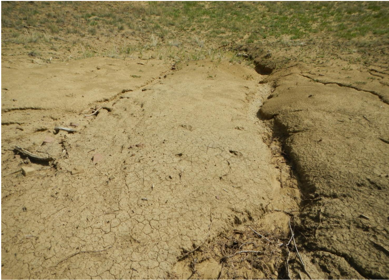
Photo 3. View of erosion and poor revegetation on cut-slope in western portion of the project area.
