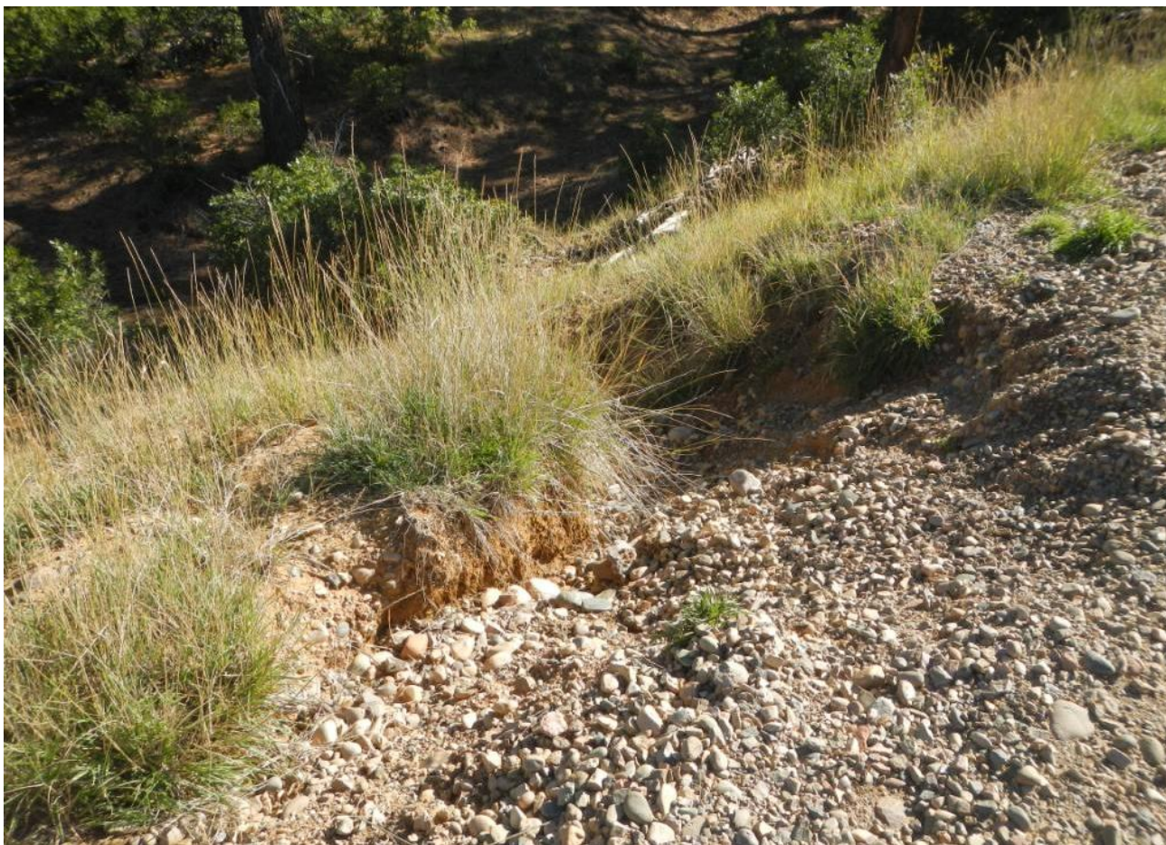
Photo 2. View of erosional channels along the steep edge of the access road near the entrance to the well pad.
