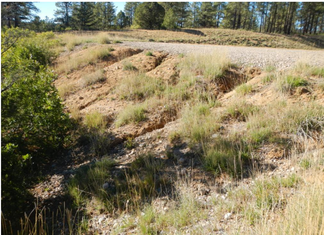
Photo 1. View of erosional channels on the southern edge of the working area of the well pad.
