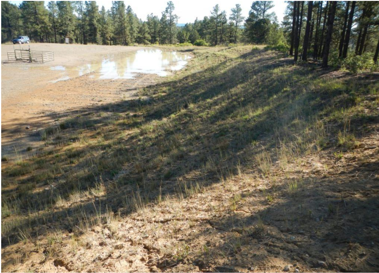
Photo 5. View of cut slope in western portion of the project area. Slope is largely stabilized with vegetation. Minor rill erosion is occurring. Large puddle appears to be contained and is primarily away from driving surfaces.
