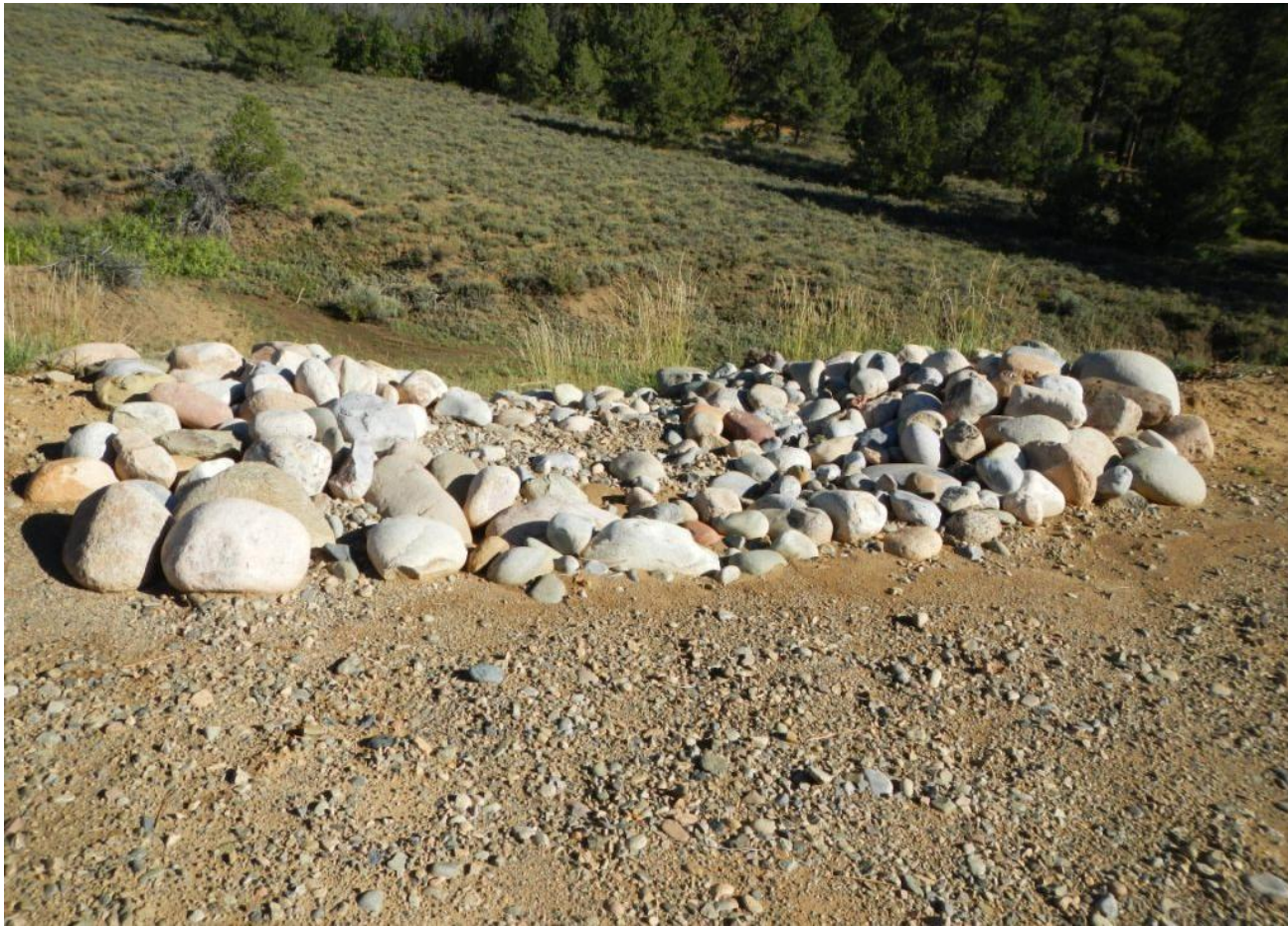
Photo 3. View of cobble BMP on the surface of the well pad that appears to be in good condition and is likely effective at de-energizing and filtering stormwater flows exiting the well pad here.
