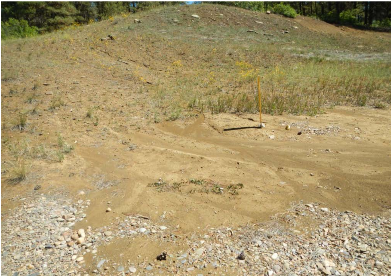
Photo 3. View of cut slope on the eastern edge of the project area. Rill erosion is occurring on the slope and sediment is running onto the well pad.
