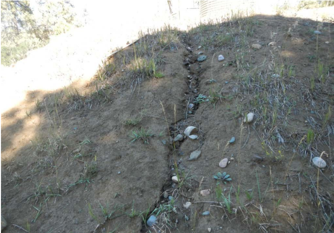
Photo 5. View of rill erosion on the southwestern corner of the project area.
