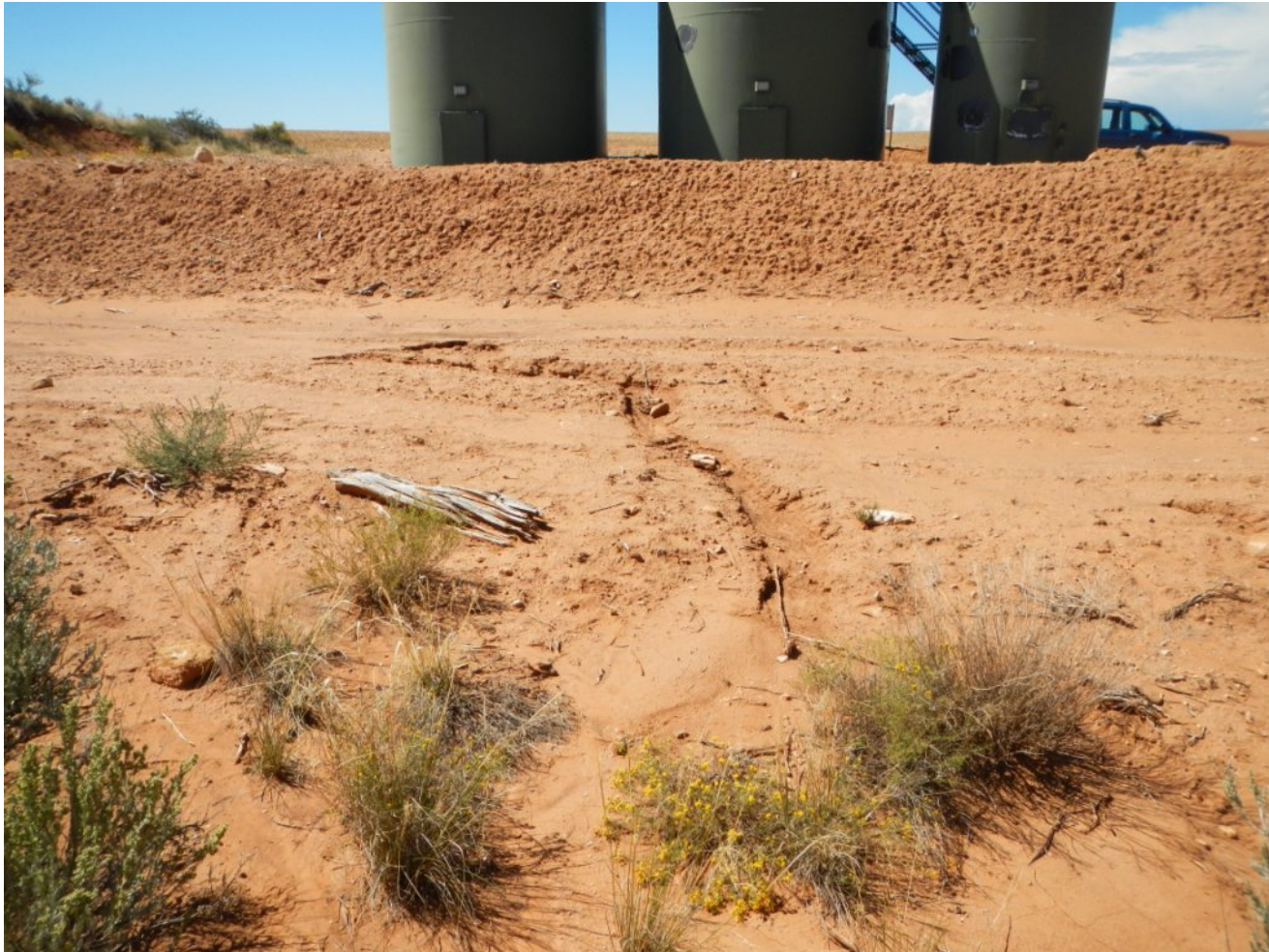
Photo 4. View of more rill erosion on eastern edge of well pad.
