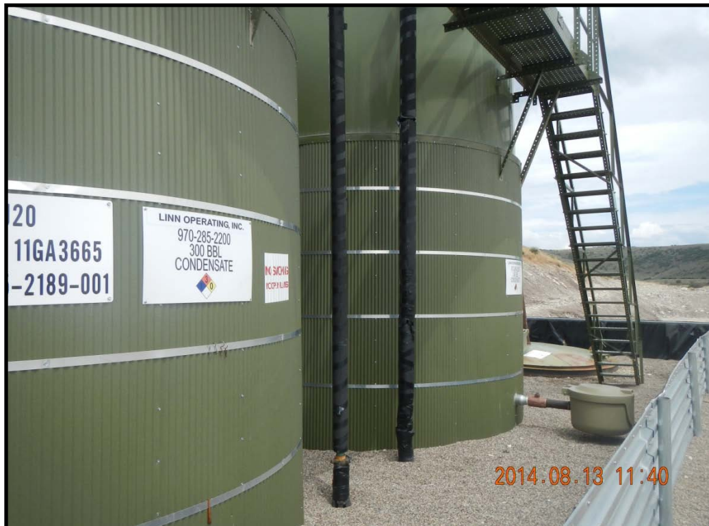
Tanks with secondary containment. Lined, clean.
