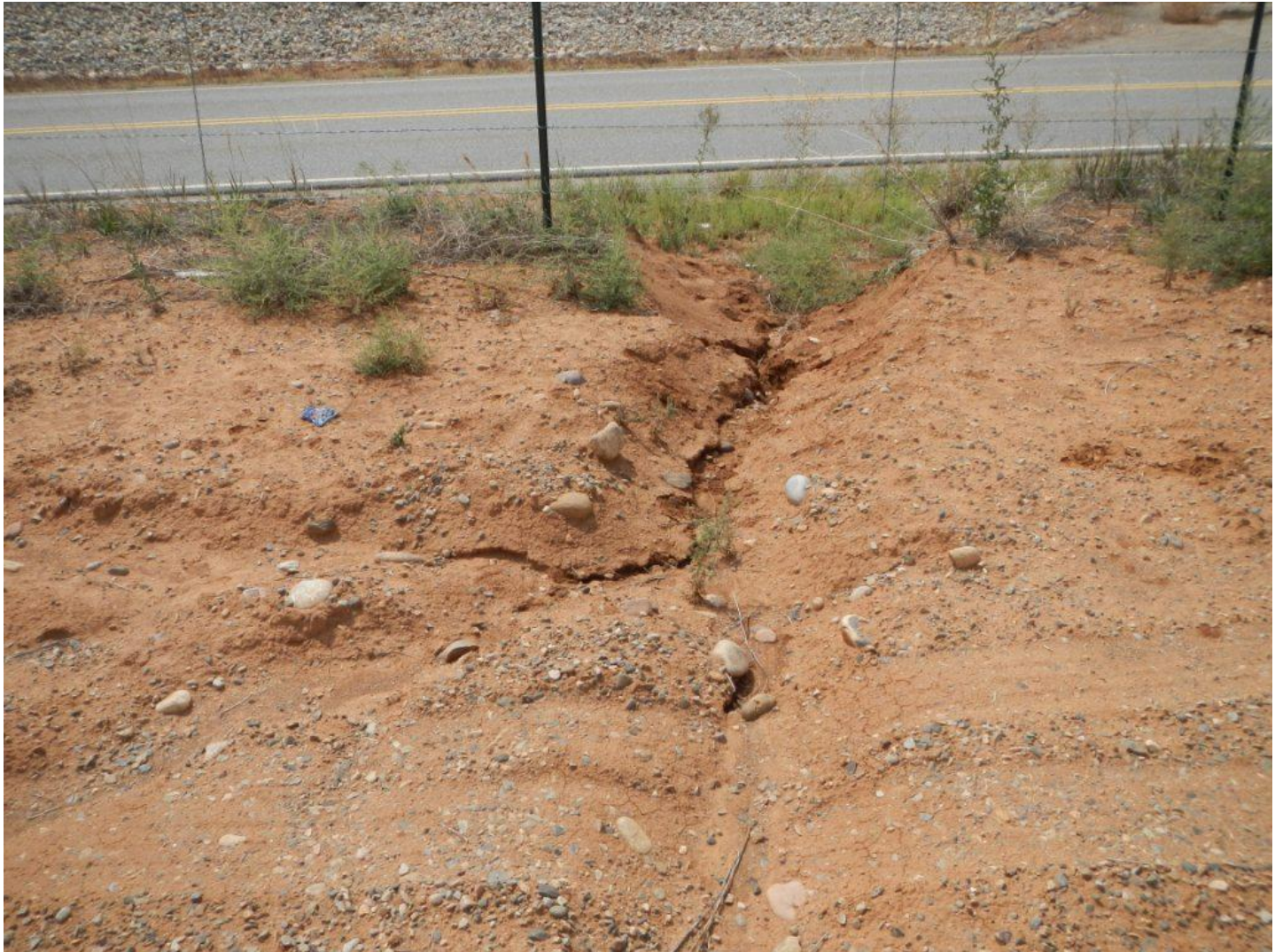
Photo 4. View of rill erosion along southern edge of well pad.
