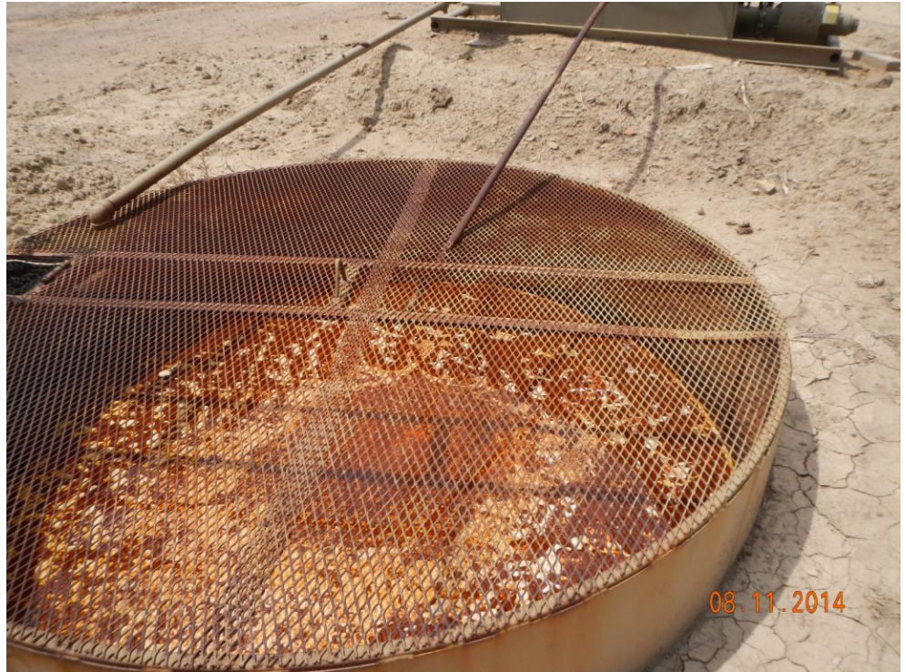
Produced water tank.
