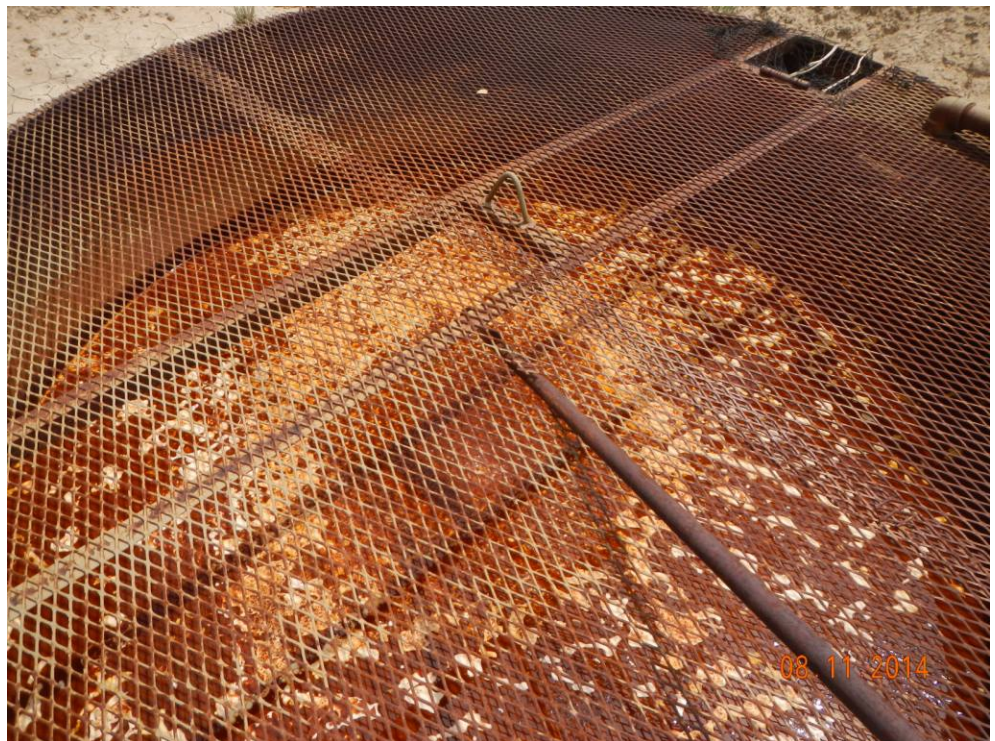
Produced water tank.
