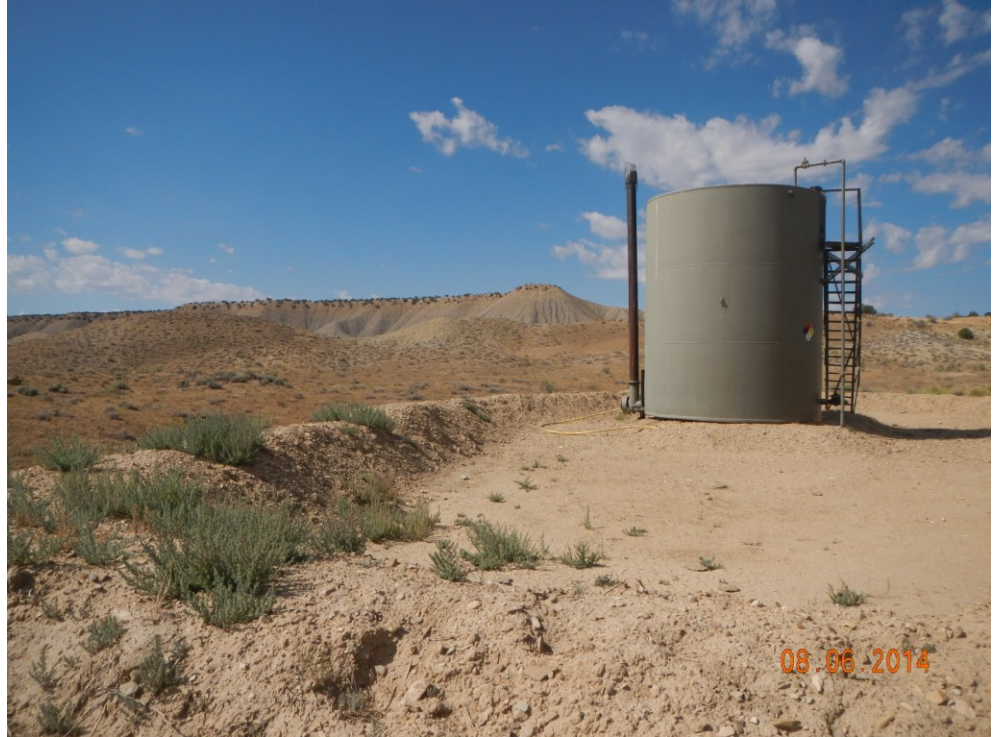
Weeds on berm and in containment.
