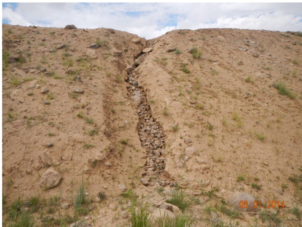
Second area of erosion on fill slope.
