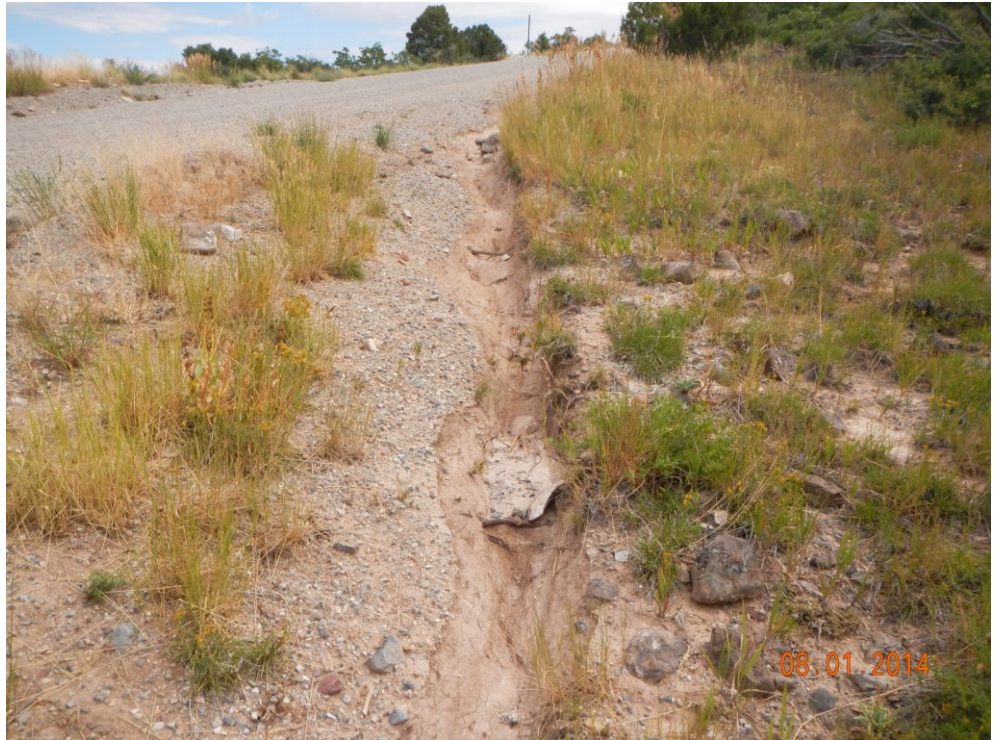
Erosion and rilling along access road.
