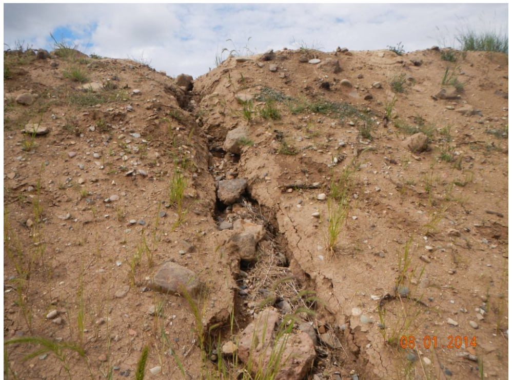
First area of erosion on fill slope.
