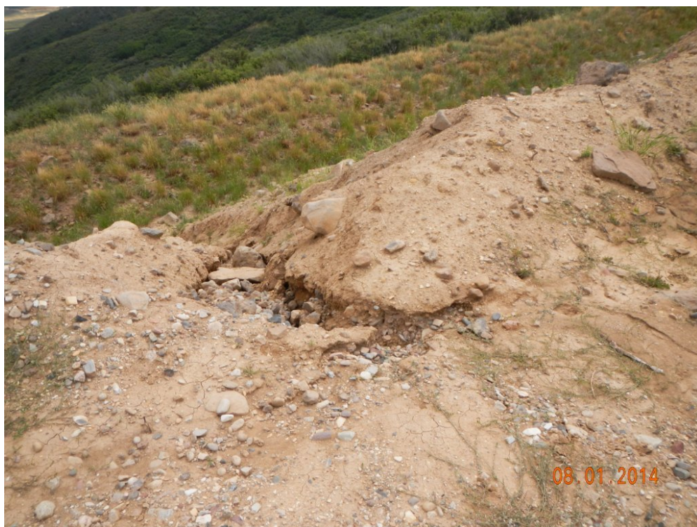
View of second area of erosion from pad.
