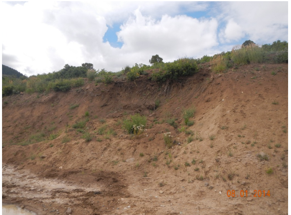
Erosion on cut slope.
