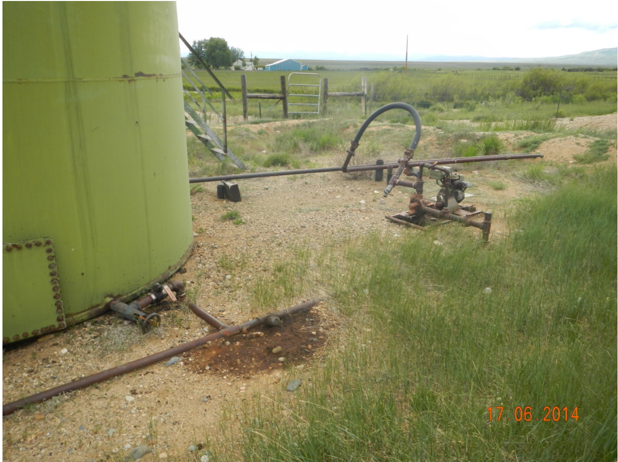
8.) Visual staining beneath oil filter.
