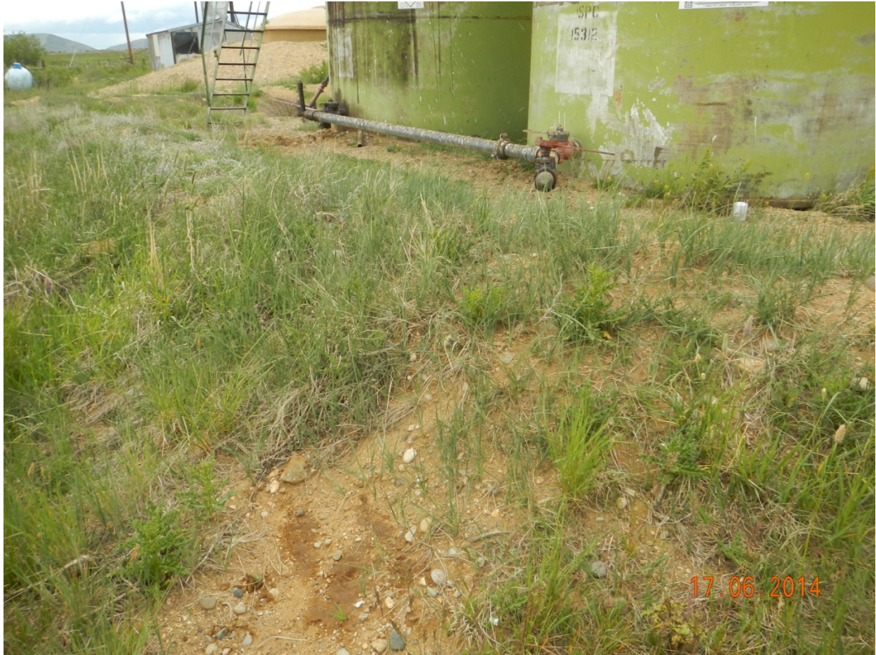
9.) Residual surface staining on berm.
