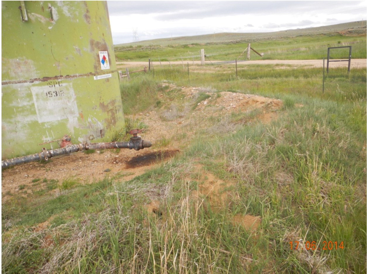
5.) Staining beneath load out valve
