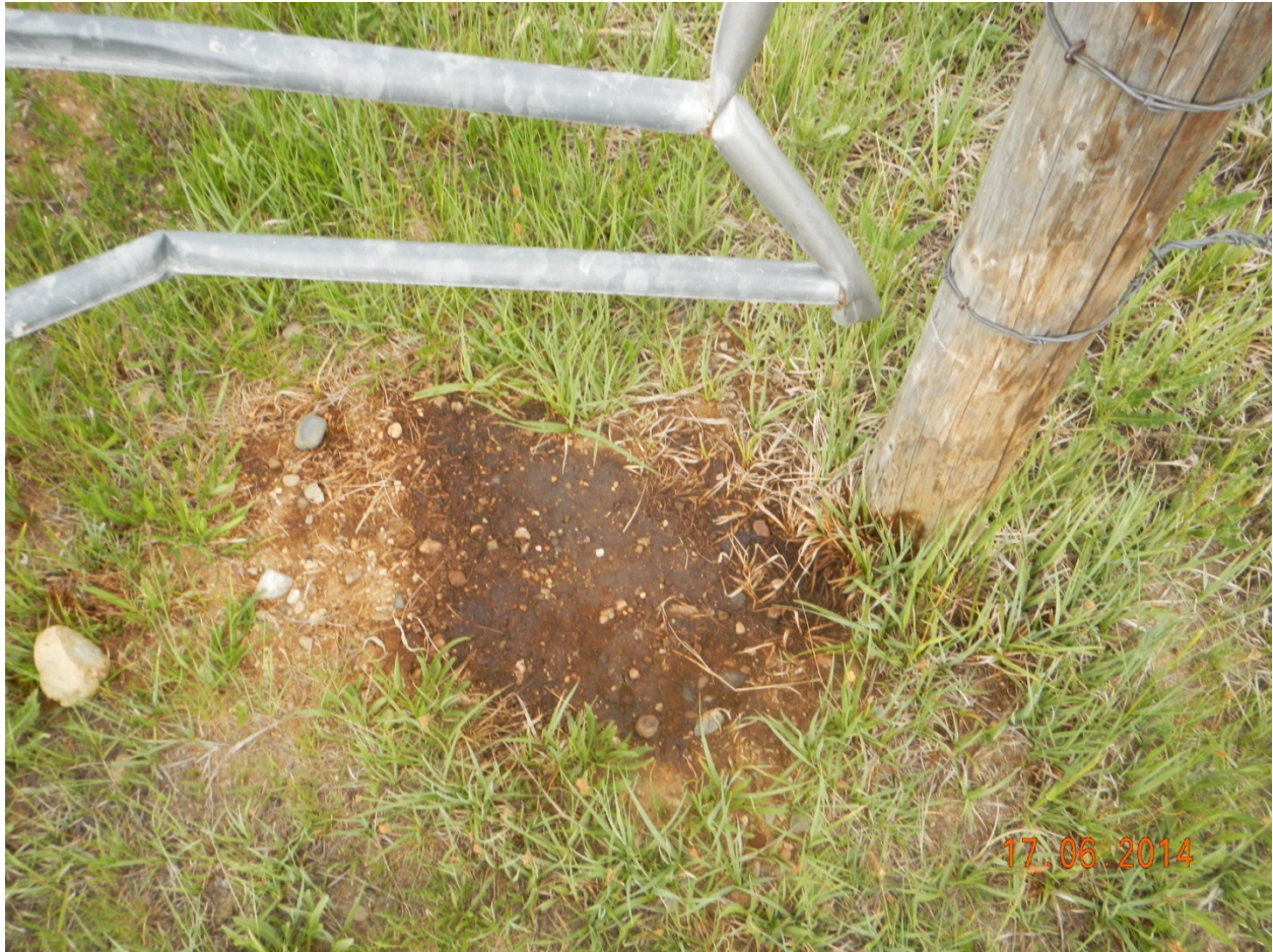
3.) Surface staining below thief hatch.
