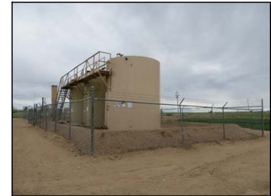
SECURITY FENCE AROUND TANK BATTERY AND PRODUCTION EQUIPMENT (TYP)
