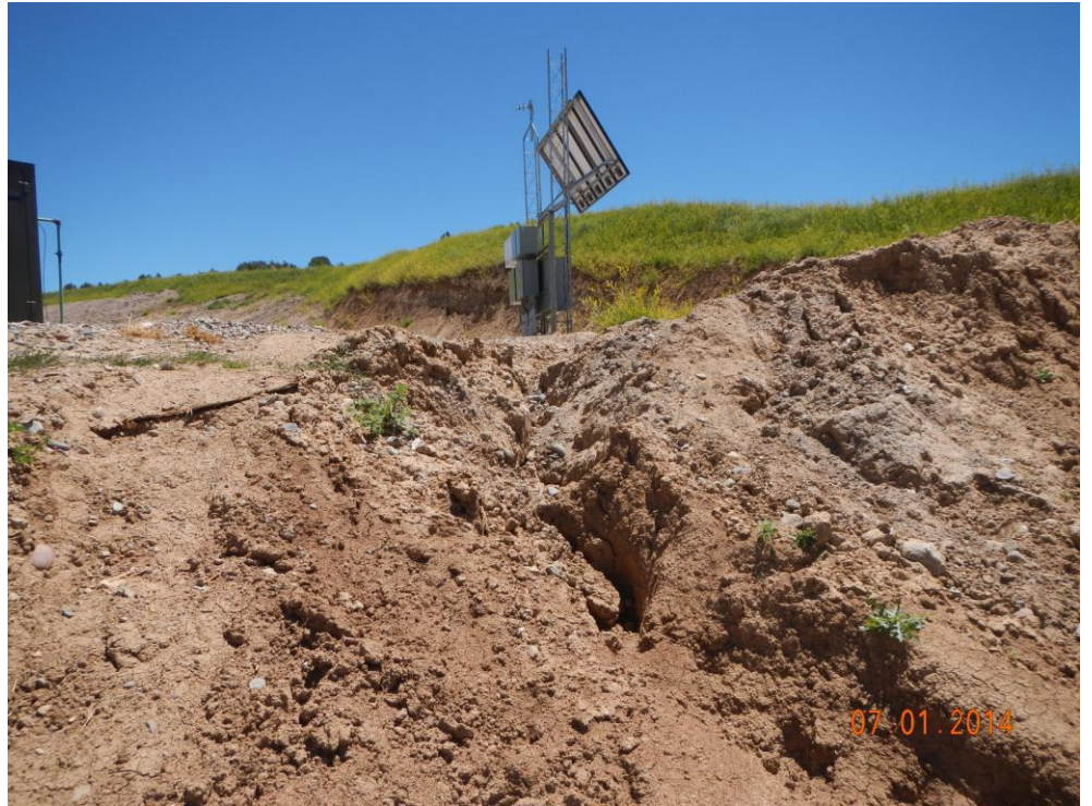
Erosion in drain area
