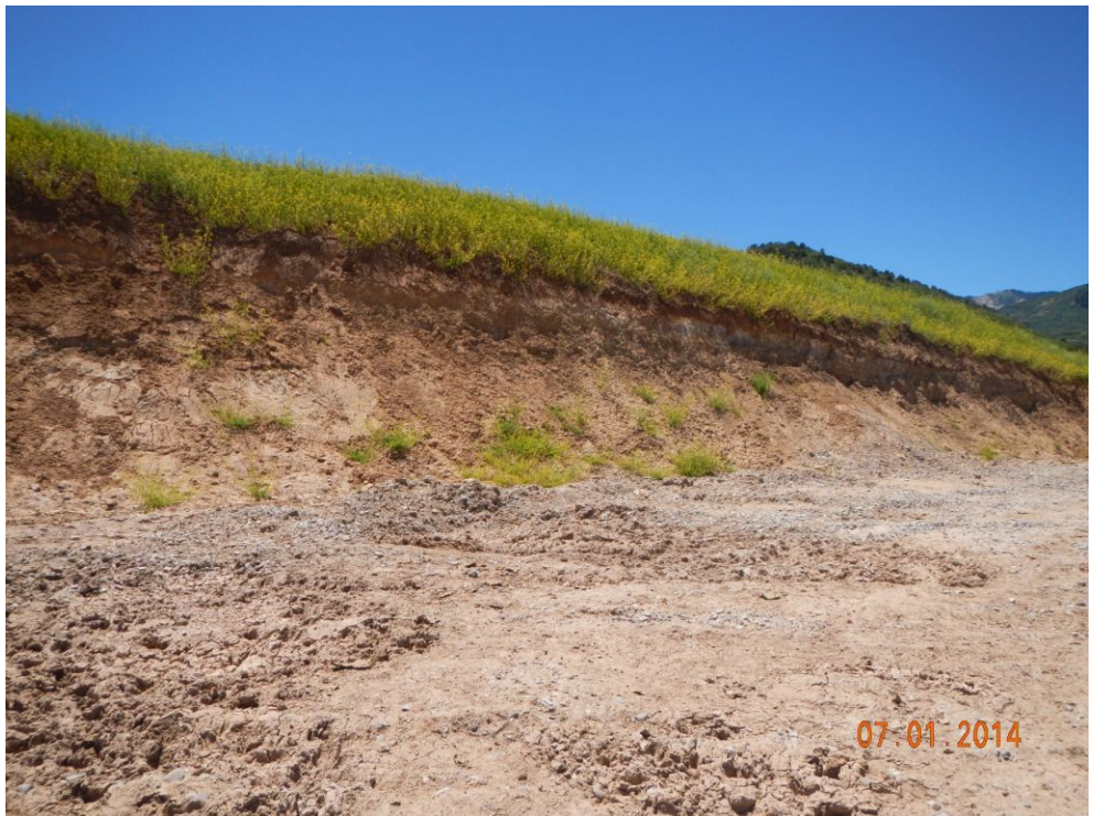
Erosion on cut slope
