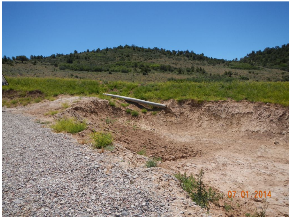
Erosion on wall of snow containment/retention pond. Unused culvert on slope.
