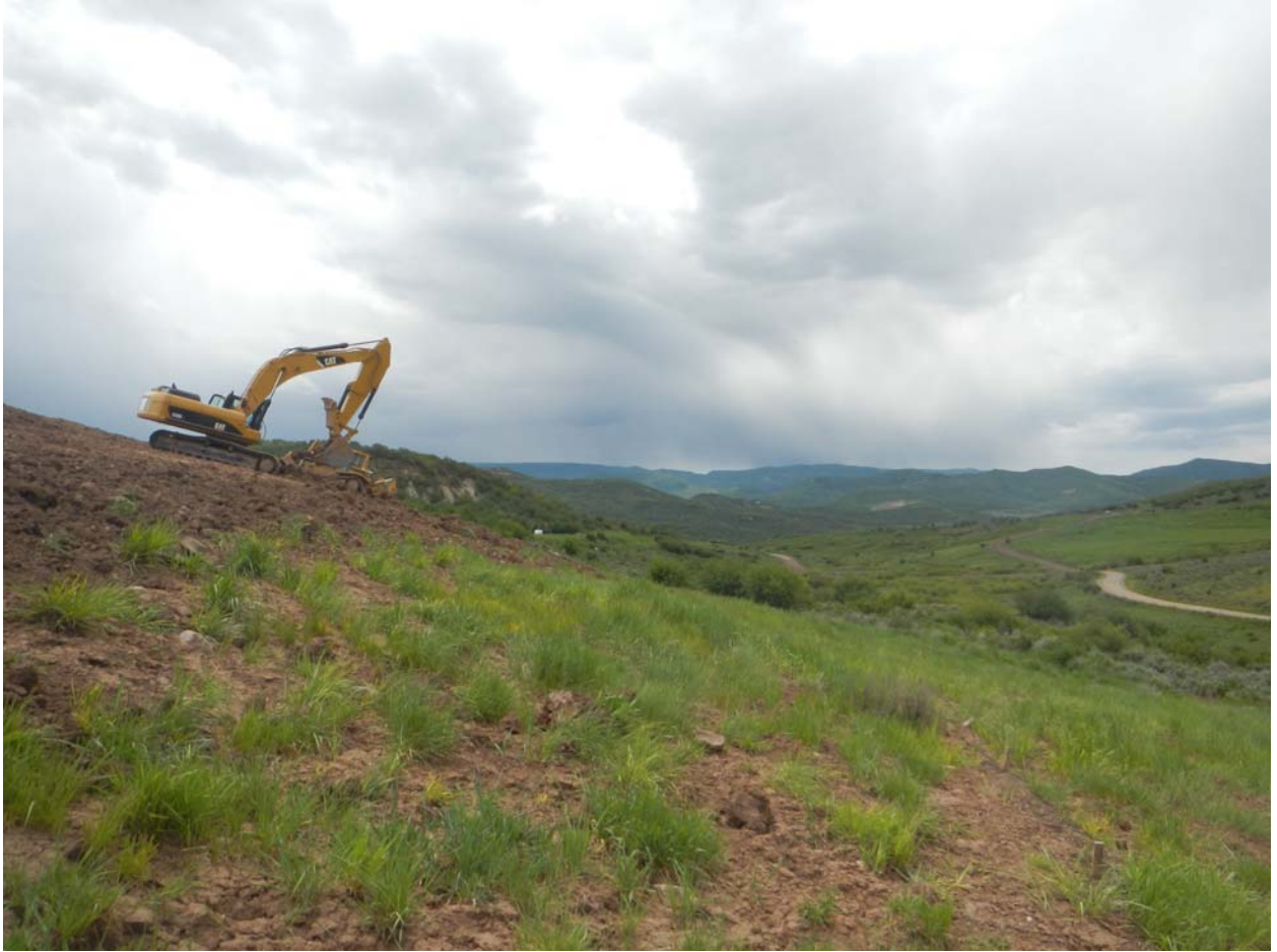
Perimeter wattles failing (2)
