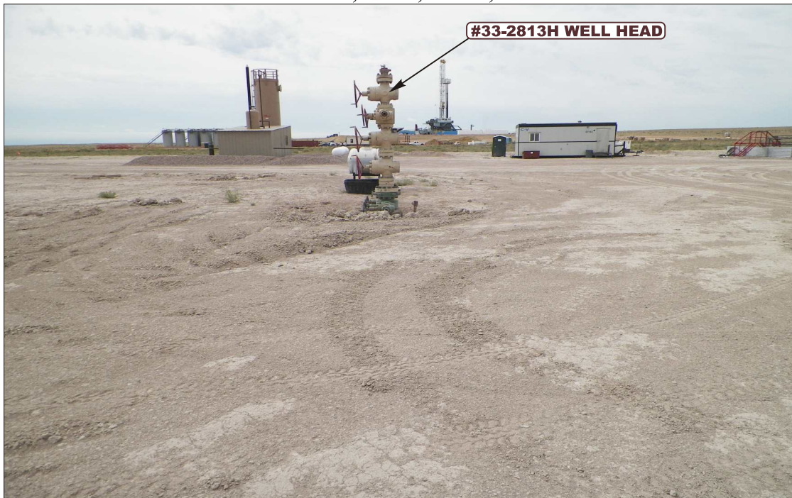
PHOTO: VIEW OF EXISTING WELL HEAD
