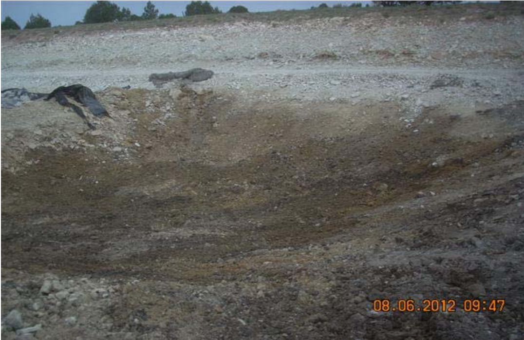
Photo 1 – View of the eastern end of the pit after removal of the liner. Photo is taken from the southeast corner looking northwest. Photo taken on 8/6/2012.
