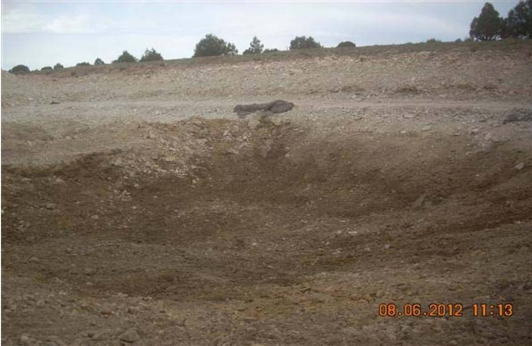
Photo 5 – View of the eastern end of the pit after removal of the contaminated soil. Photo is taken from the southwest corner looking northeast. Photo taken on 8/6/2012.
