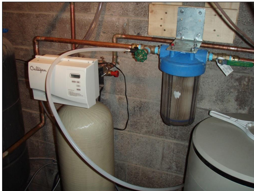
Photo 2. Puckett Well Sampling Location (GM 323-28-151879 & 172632-dup); Point Before Softener
