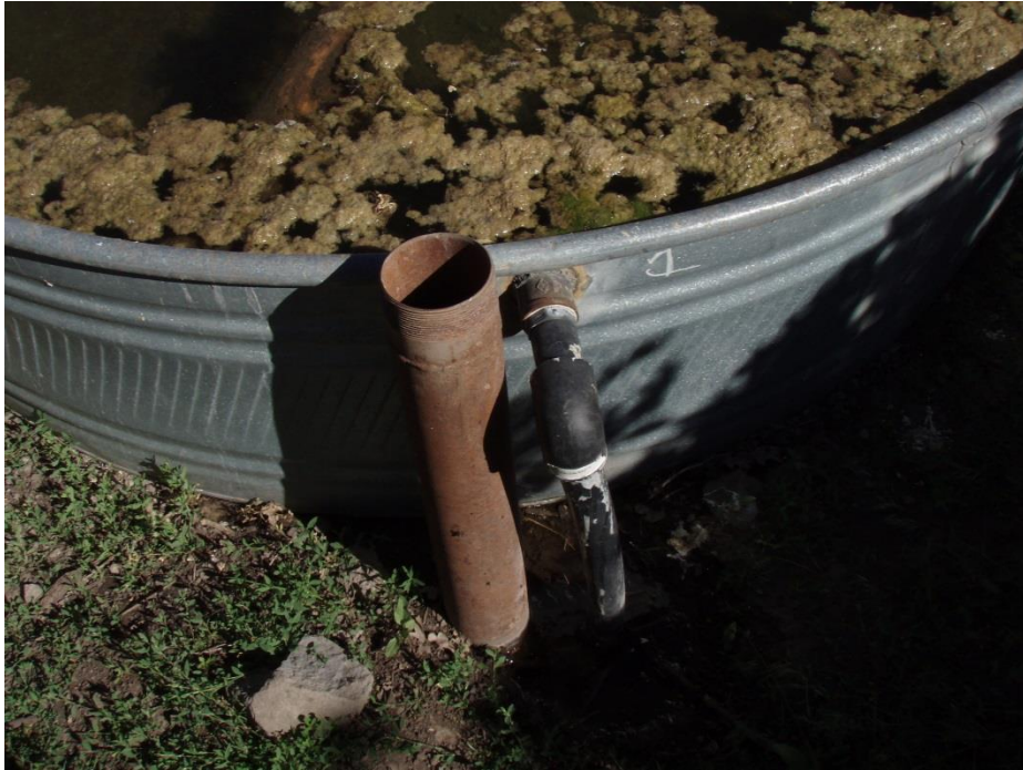
Photo 3. Yellow Jacket Spring; Second Pipe Plumbing to Stock Watering Tanks
