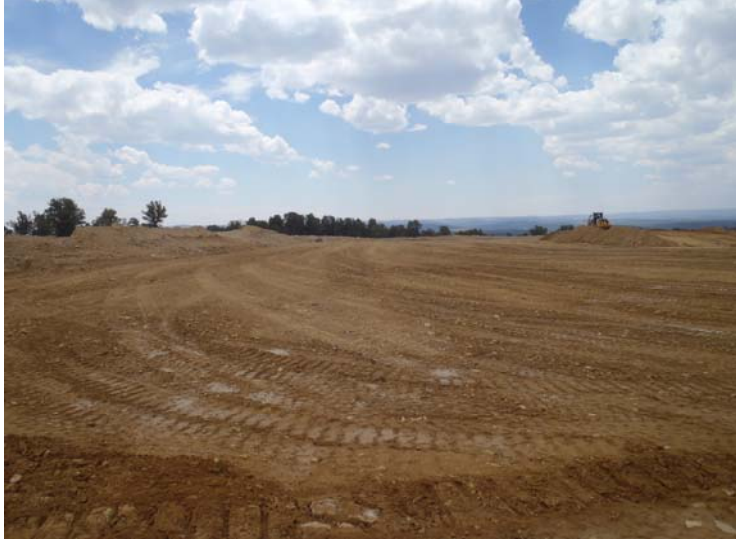
Photograph 1 – View of completed pit closure, SE side facing SW, closed Cuttings Pit
