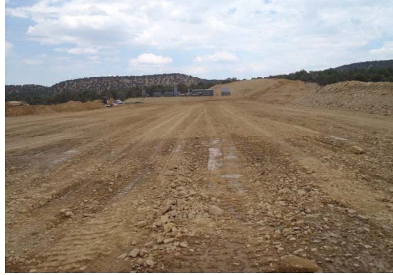
Photograph 2 – View of completed pit closure, W side facing E, closed Cuttings, Reserve and Freshwater Pits
