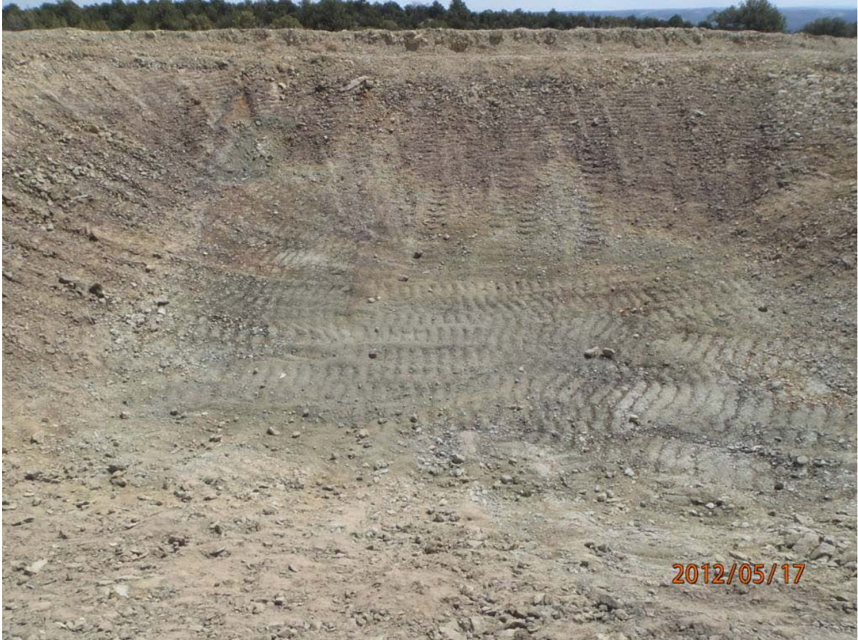
Visual representation of the impacted soils on pit bottom and pit walls prior to excavation
