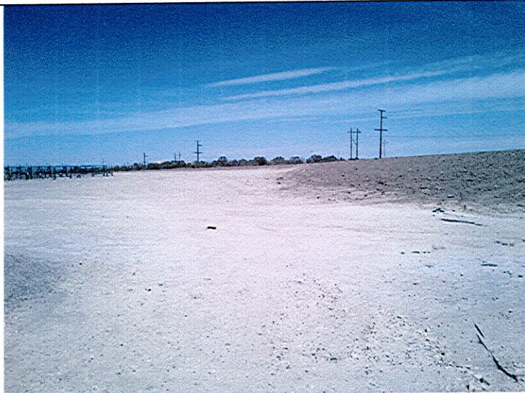
Photograph 1 – View of completed pit closure; Cuttings pits, Freshwater and Reserve Pits, photo taken 10/5/2012, S side facing N
