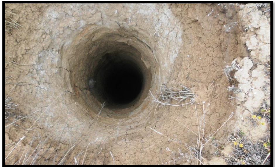
>2' dia. open borehole, estimated at approx. 20'. No groundwater or fluid was observed in the borehole @ the time of inspection.
