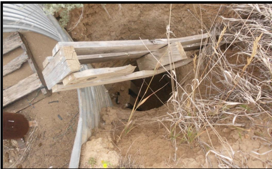
Partially caved-in (filled) rathole.
