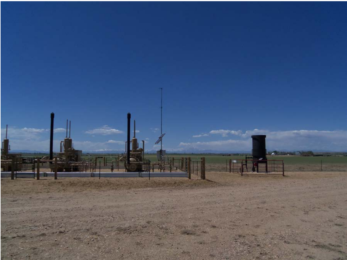
CANNON TANK BATTERY 36N-W3HZ
