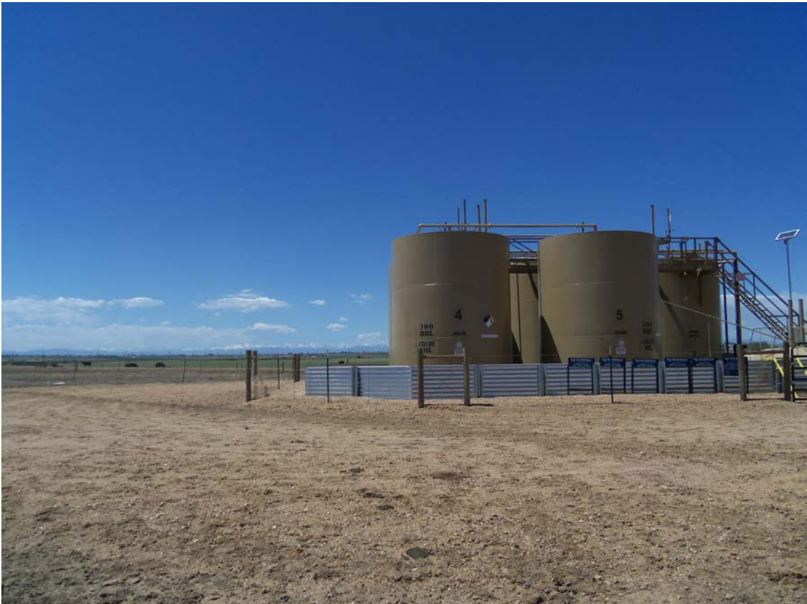
CANNON TANK BATTERY 36N-W3HZ
