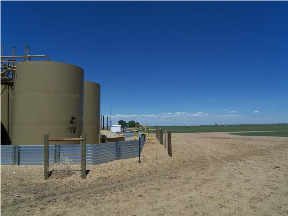
CANNON TANK BATTERY 36N-W3HZ
