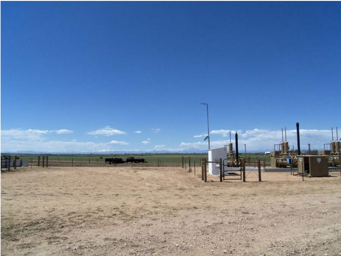
CANNON TANK BATTERY 36N-W3HZ
