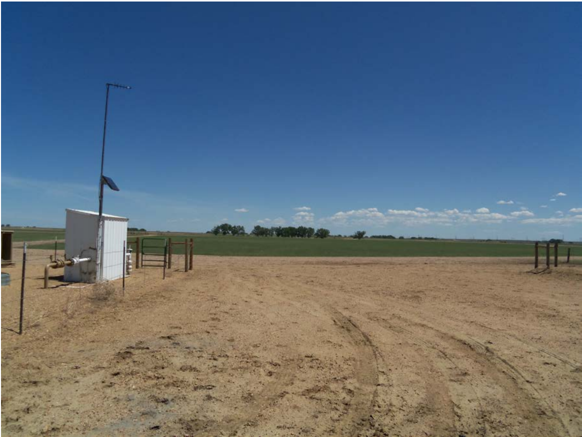
CANNON TANK BATTERY 36N-W3HZ
