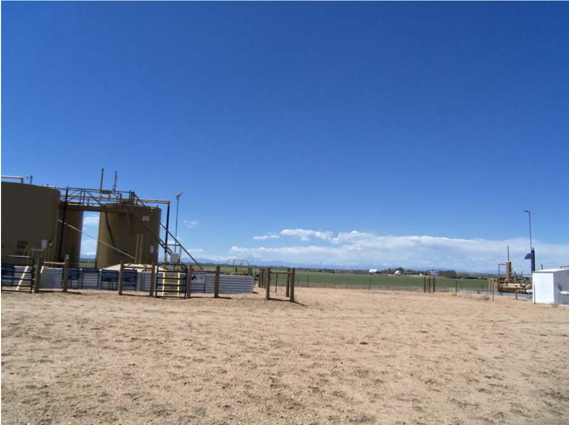
CANNON TANK BATTERY 36N-W3HZ
