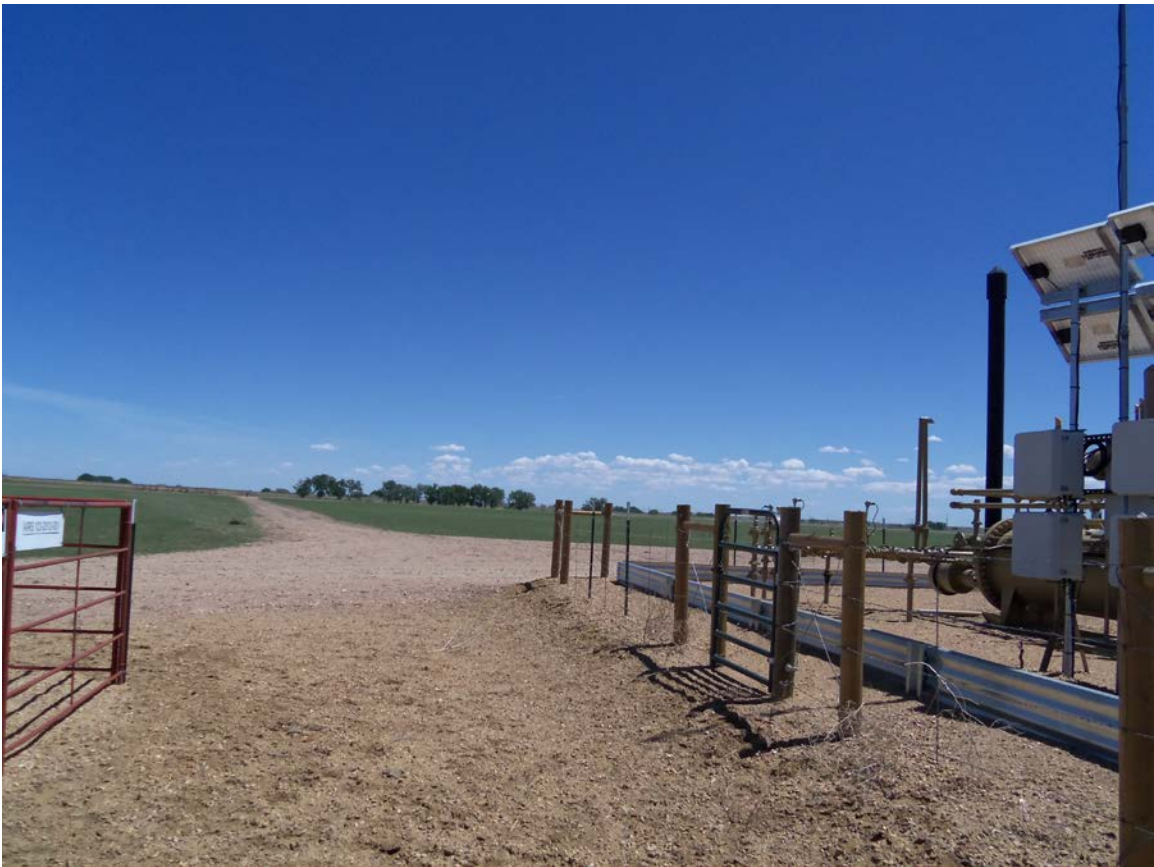
CANNON TANK BATTERY 36N-W3HZ
