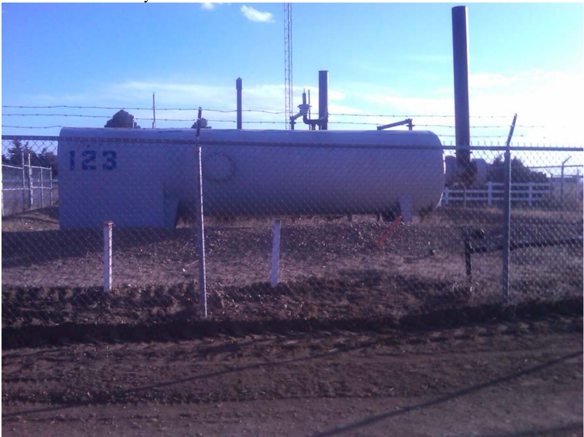
Overlook Tank Battery 27-30
