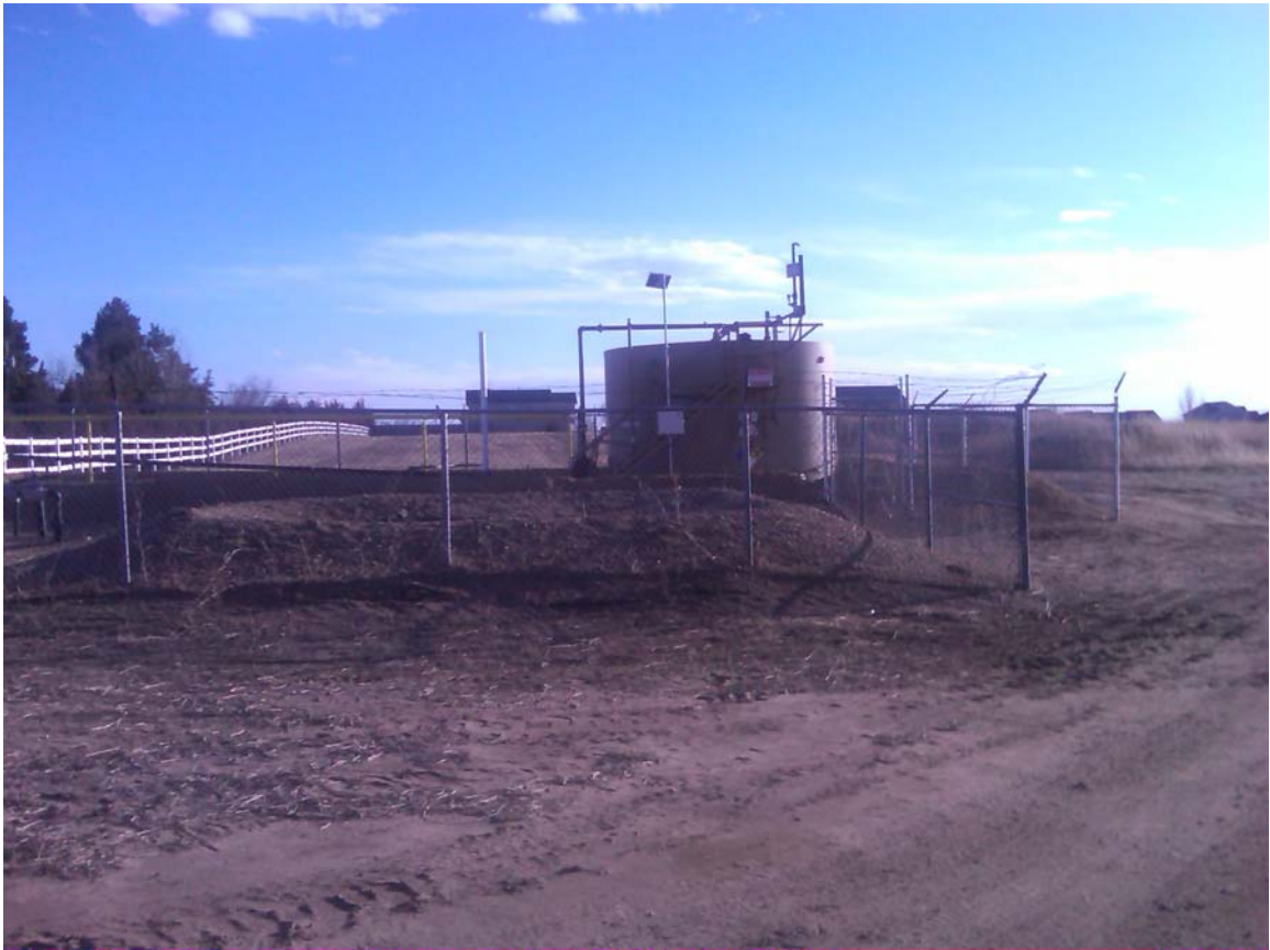
Overlook Tank Battery 27-30
