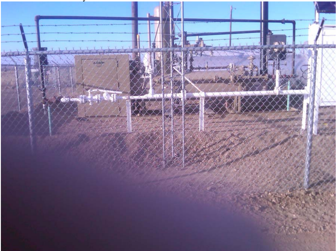
Overlook Tank Battery 27-30
