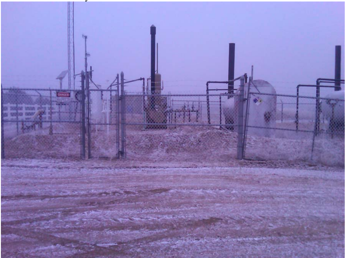
Overlook Tank Battery 27-30
