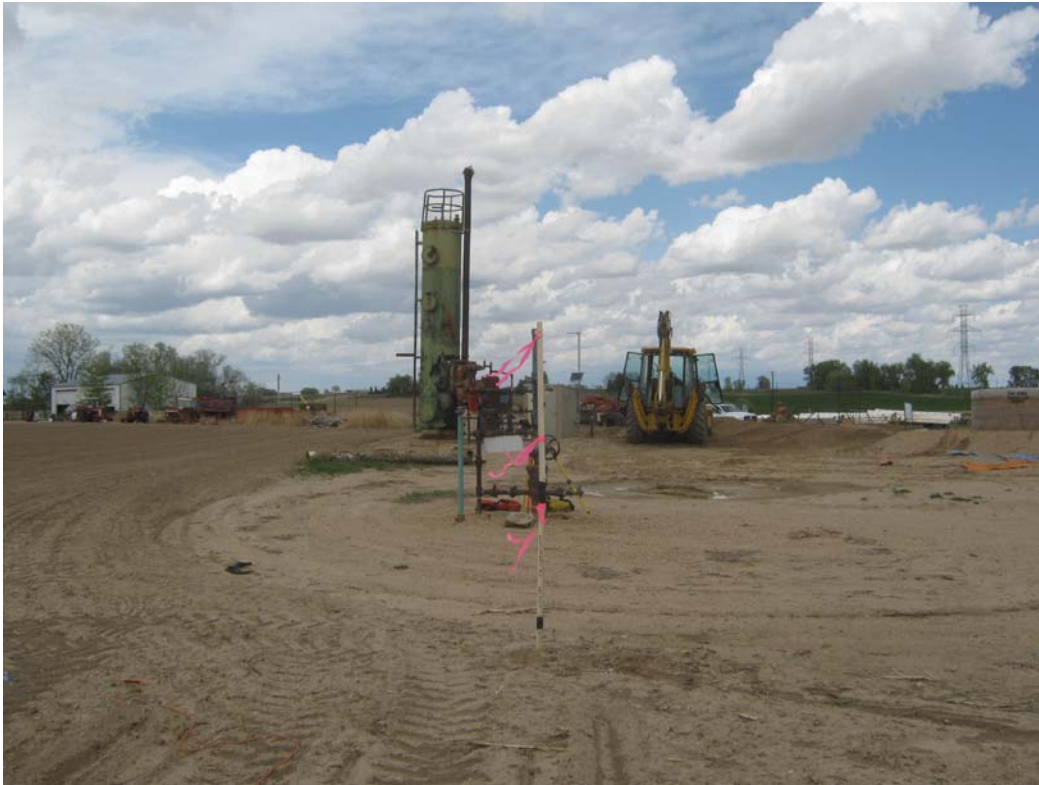
North Poudre 2-30 looking North
