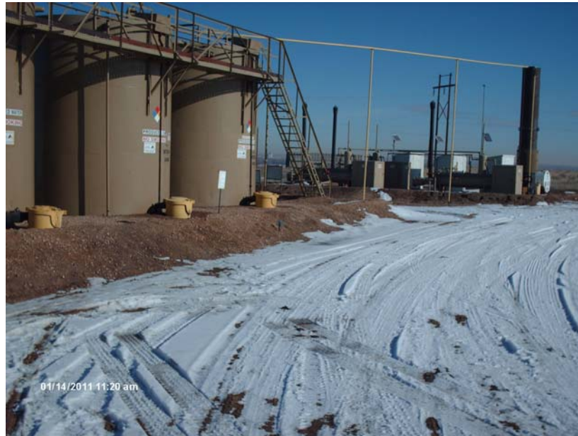
WETCO FARMS 23-4 TANK BATTERY SITE NE SW1/4 SEC. 4 T4N R63W LOOKING SOUTHEAST JANUARY 14, 2011
