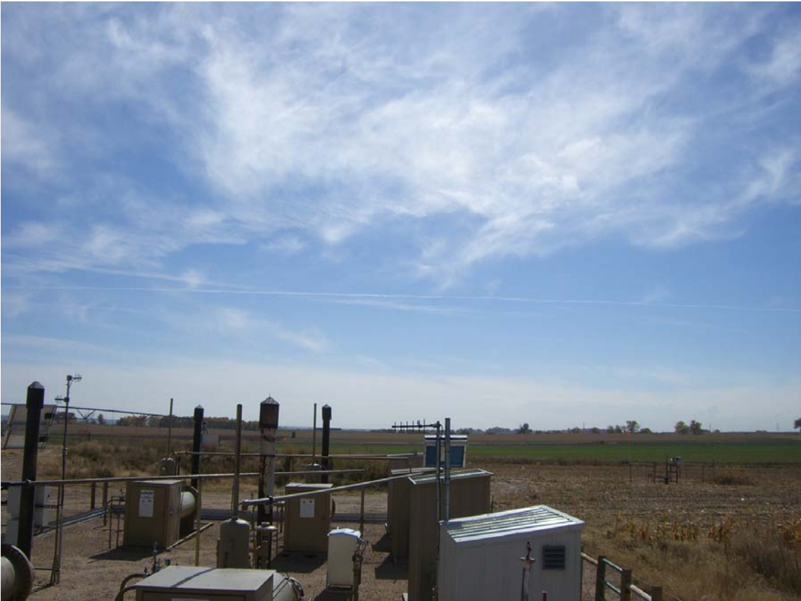
Warner Tank Battery 33-18
