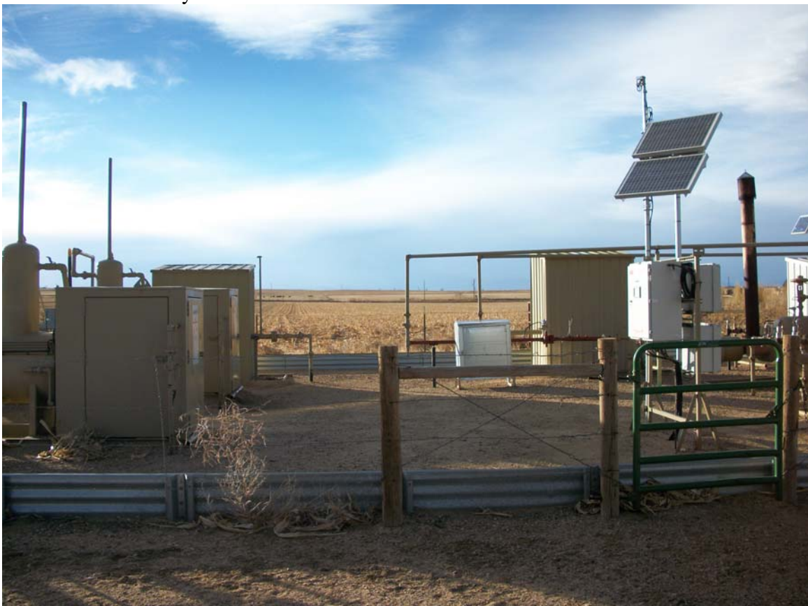
Warner Tank Battery 33-18
