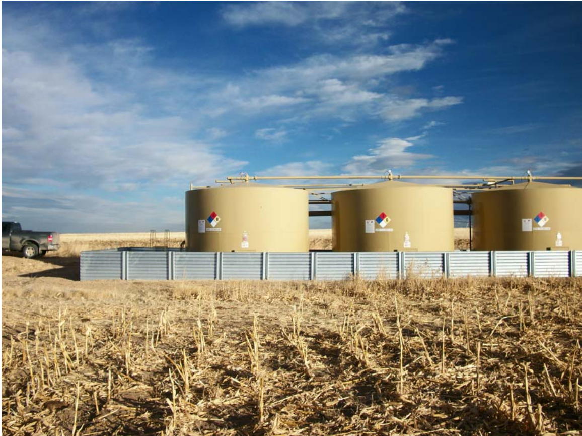
Warner Tank Battery 33-18
