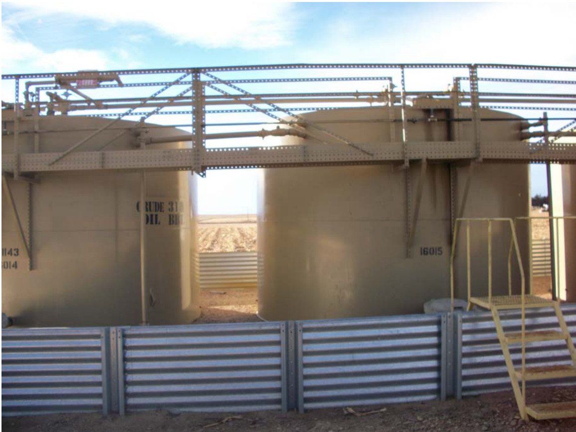
Warner Tank Battery 33-18
