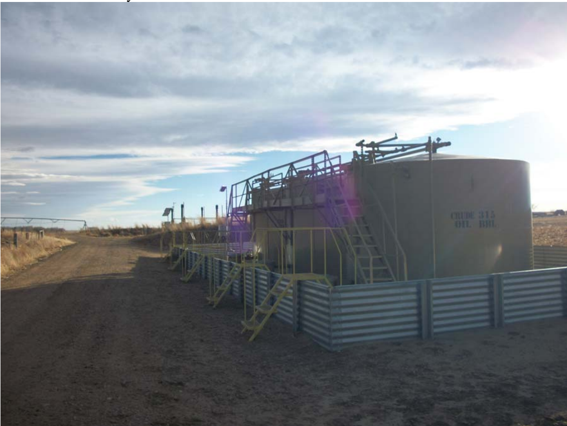
Warner Tank Battery 33-18
