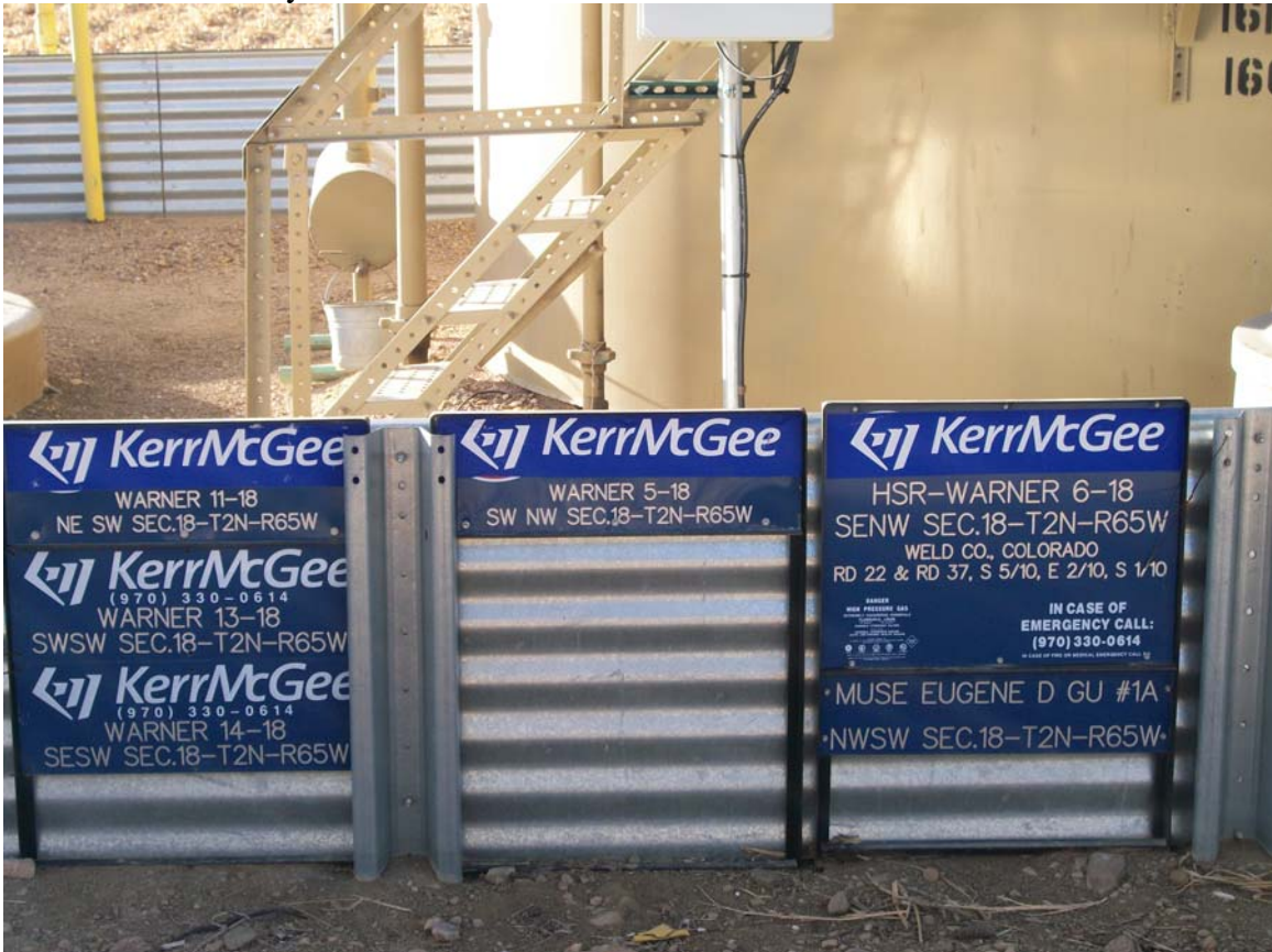
Warner Tank Battery 33-18
