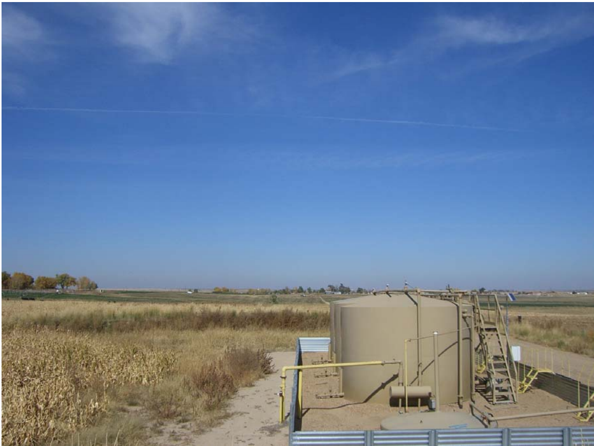
Warner Tank Battery 33-18 Location North NWSW Section 18-2N-65W 12/10/10
