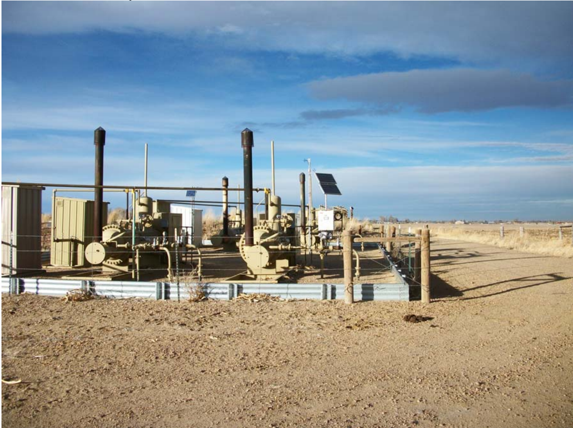
Warner Tank Battery 33-18
