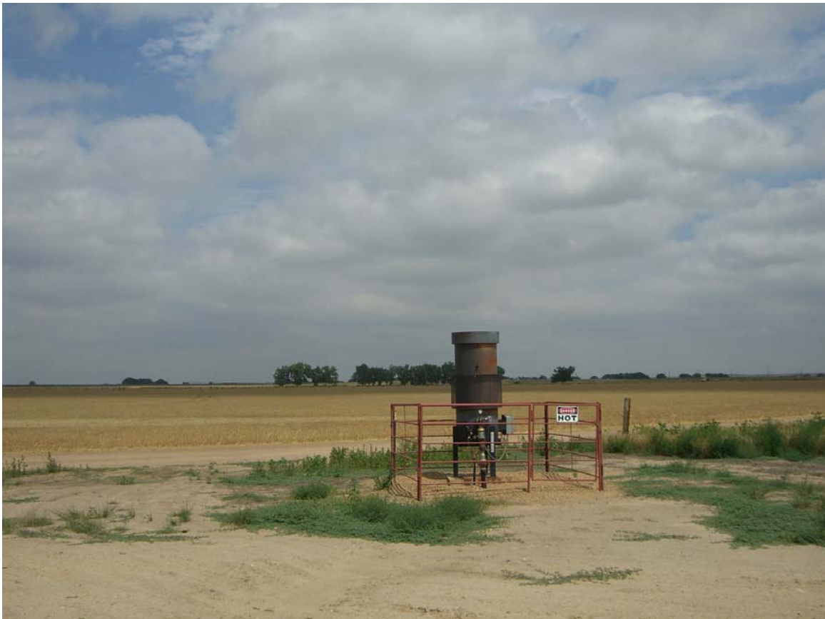
Cannon Tank Battery 24-3
