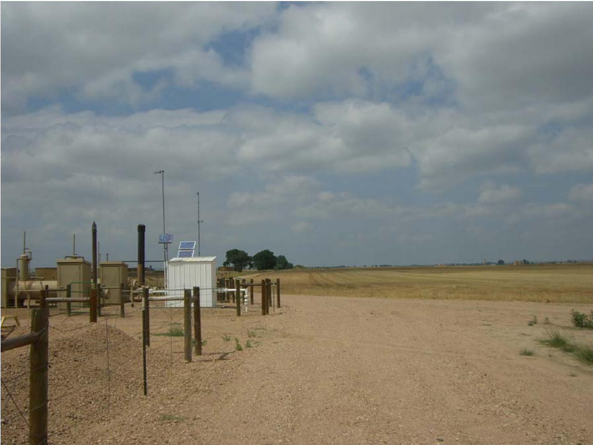
Cannon Tank Battery 24-3 Location North SWNE Section 3-2N-65W 07/20/10
